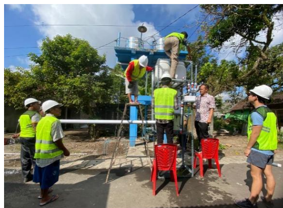
The caretaker of the communal SPAM in Kedungsari village installed a hydrochlorination system on 26 May 2023.
