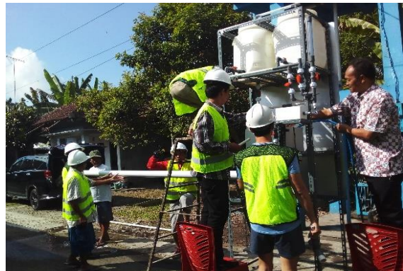
The pilot project of hydrodoser installation in the communal water supply system (SPAM) in RT3/RW6 in Kedungsari urban village, North Magelang sub-district, Magelang city. The installation takes place from May 23 rd to 25 th , 2023 and involves the communal SPAM caretaker group. W6.
