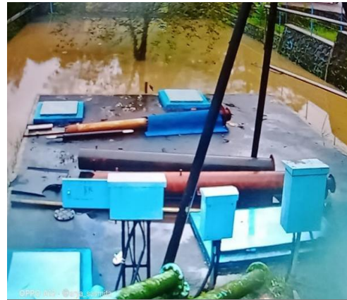
Damage to Broncapturing Tuk Pecah (Intake) assets due to flash floods at PDAM Magelang City, causing the service to stop for several days.
