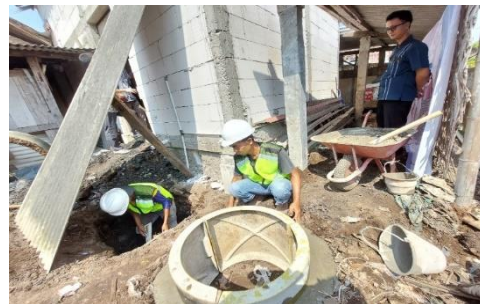
Training and Practice in Building SNI Standard Septic tanks included in the Negative Determination with condition (NDWC) category, wherein the training provides understanding of safety work and mitigation of potentially dangerous activities.
